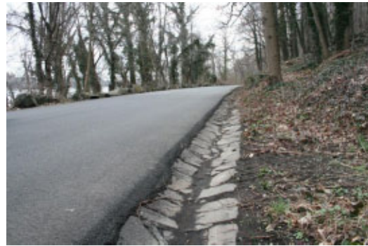
Existing photo of the stone gutter along Henry Hudson Drive. Note the raised asphalt surface.
