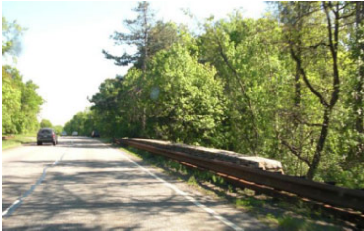
Photo of the metal guide rails in front of the original parapet wall on the New Jersey section of the Palisades Interstate Parkway
