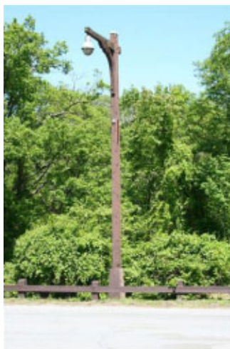
Existing light at Bear Mountain parking lot
