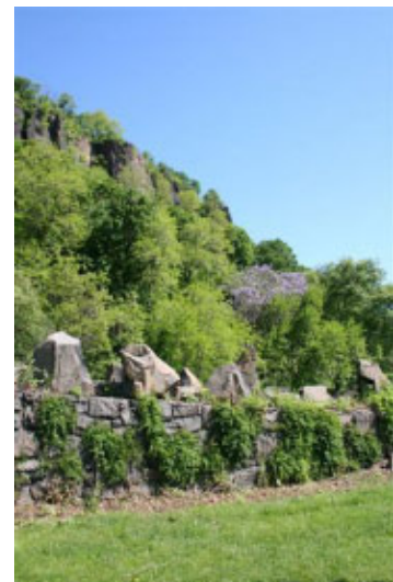
Invasive plant material attached to parapet wall
